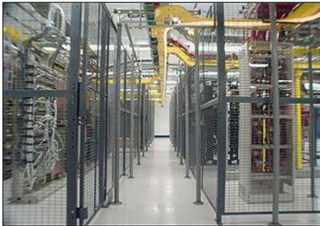
Figure 3 – Server Security Cages
